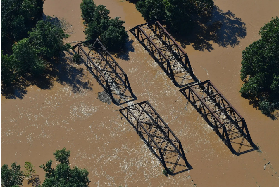
Figure 15 : Bridge in Somerset County Inundated by Floodwaters
